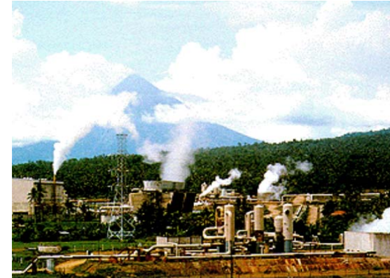
Tiwi Geothermal Power Plant Complex
